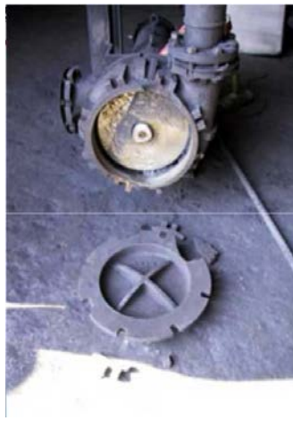
Pump Exploded Causing Fatality
