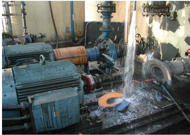
Duty Pump with ‘Remains’ of Standby Pump
