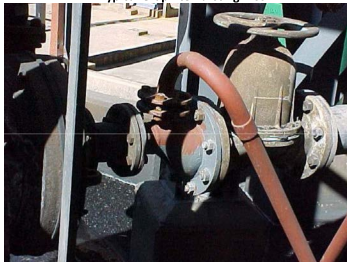
Bursting Disc Installed
