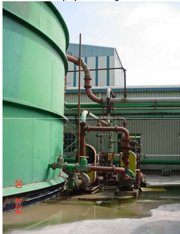
Standby Pipe Directly Vertical
