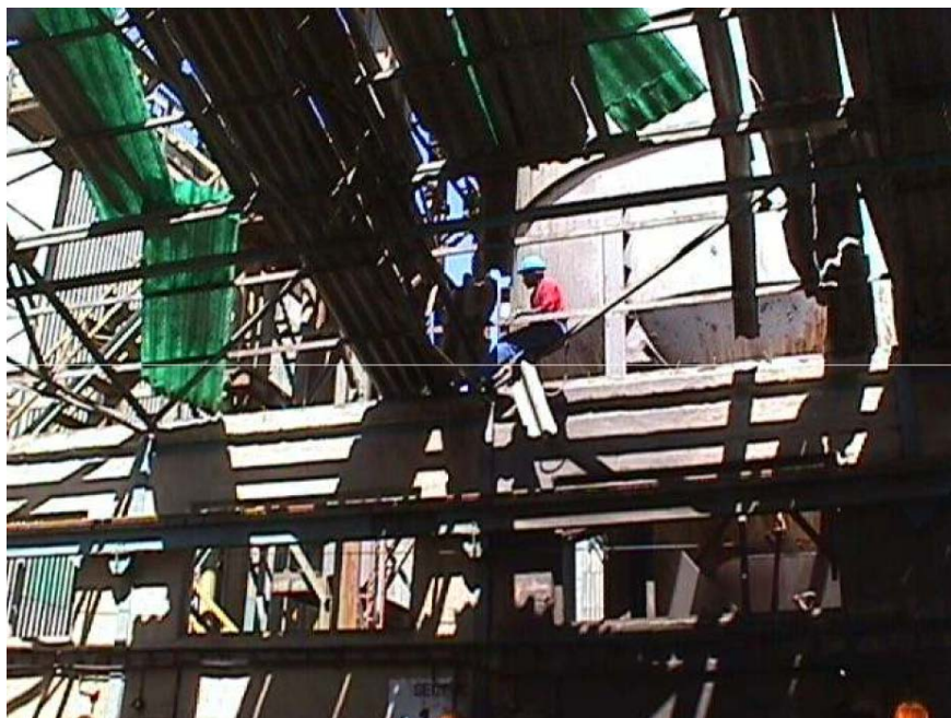
Roof Damaged by 14/12 Explosion
