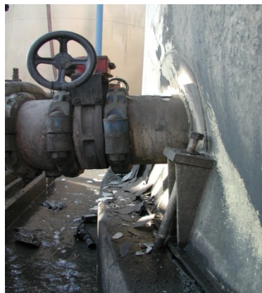
Suction Tank and Piping Bent
